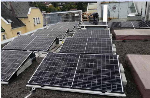
Neue Photovoltaikanlage, RGS Landeck, Foto: AMS
